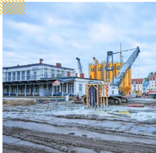
Ludwigslust, Germany: Implenia is carrying out special foundations work for the new railway bridge.
